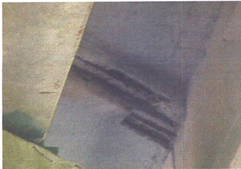
SPAN #2 EXPOSED REBAR BETWEEN 'C' AND 'D'
